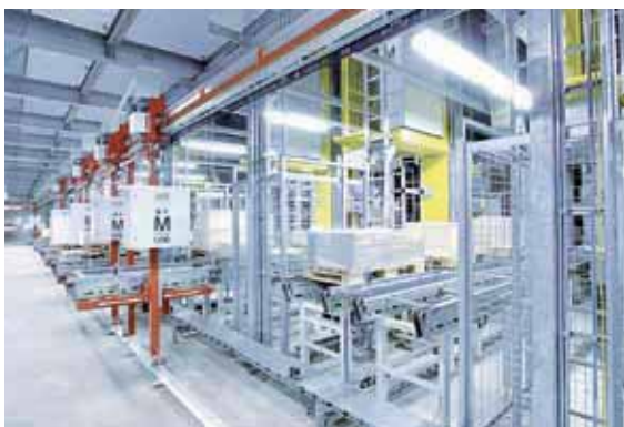
Monorail from Kardex Mlog with individual driven chassis. Modular construction with high payload and conveying speeds up to 2 m/s.
